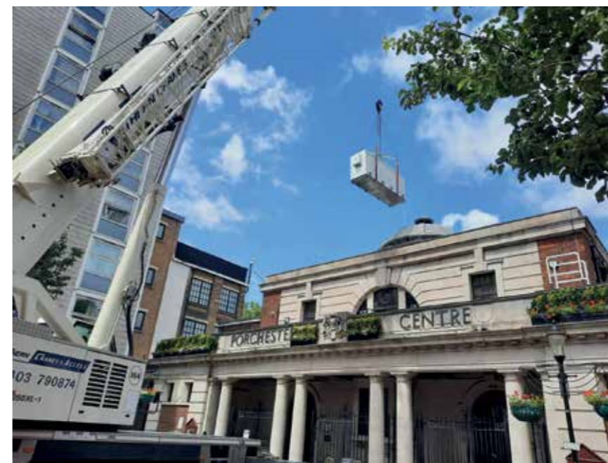
ASHP being crane lifted to the roof of a Westminster City Council building
